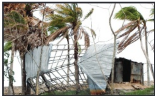
The wind is blowing the roof away.
