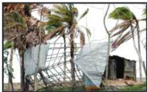
The wind is blowing the roof away.
